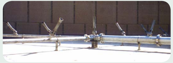
Jet Mixing System in tank
